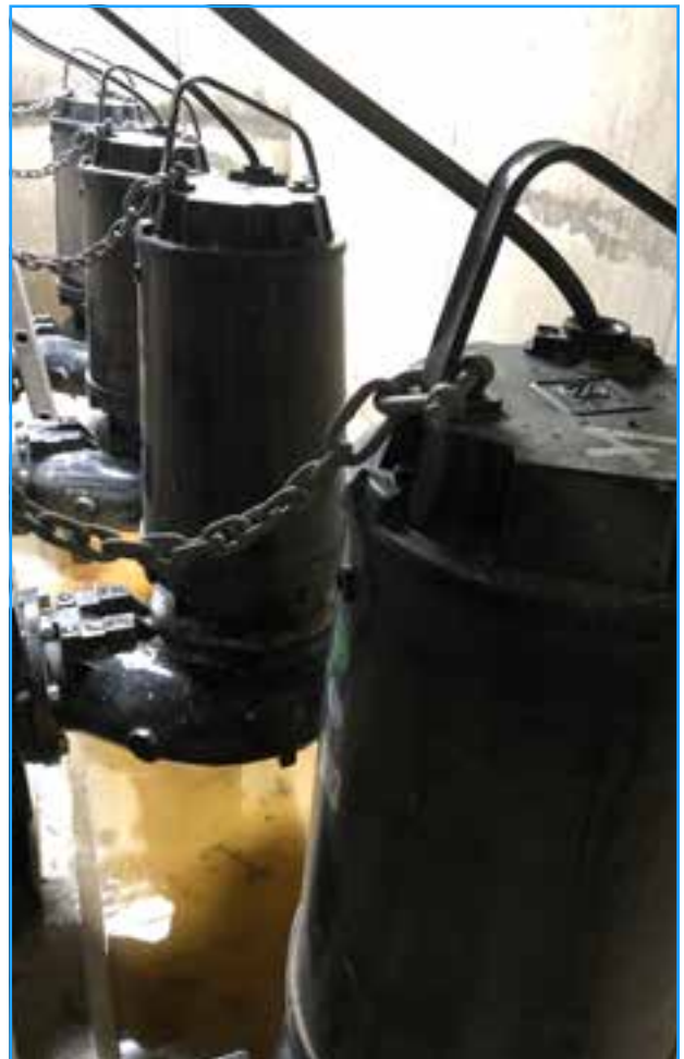
La station de pompage Uniqa.
